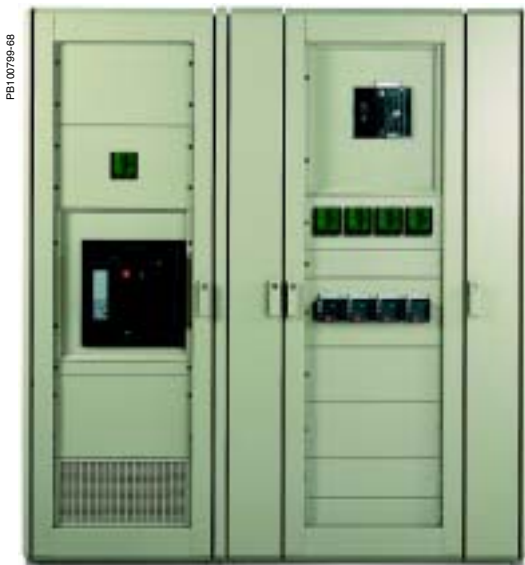
Main LV switchboard.
