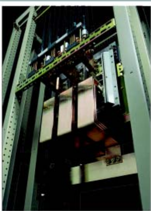
Connection to busbars.
